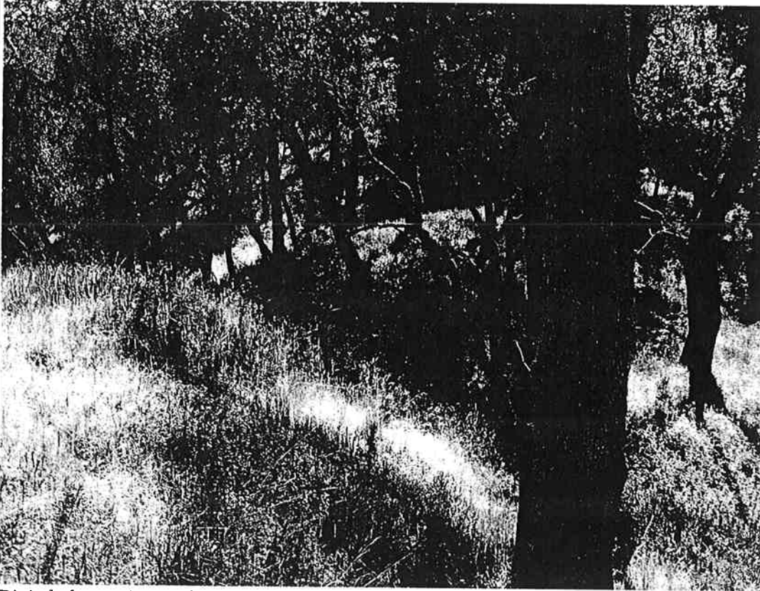
Digital photo; view to the southeast, earthen dam with breach in it.
