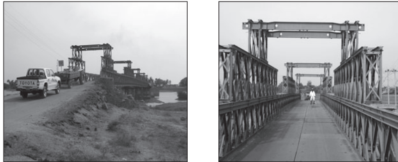
Figure 5: Temporary Bridge Currently Spanning Arugam Bay near Site of Planned USAID-Funded Bridge in Sri Lanka
