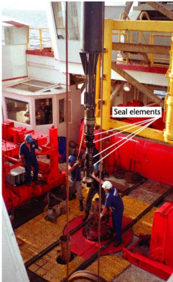
Figure 2. Lower portion of CORK with seal elements being prepared for installation in the reentry cone.
