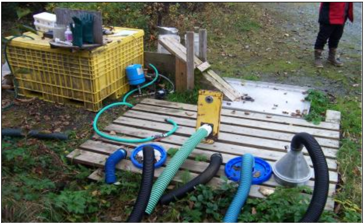
Figure 3. Existing Sewage Dump Station. This facility does not meet state DEC regulations.
