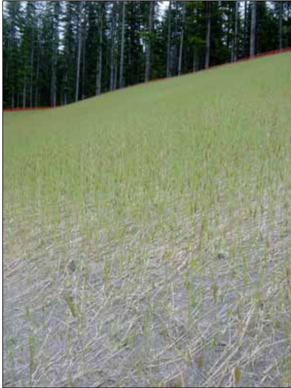
Figure 28 – Wheat hybrid grass was seeded on the slopes near the new maintenance facility to stabilize the soil.
