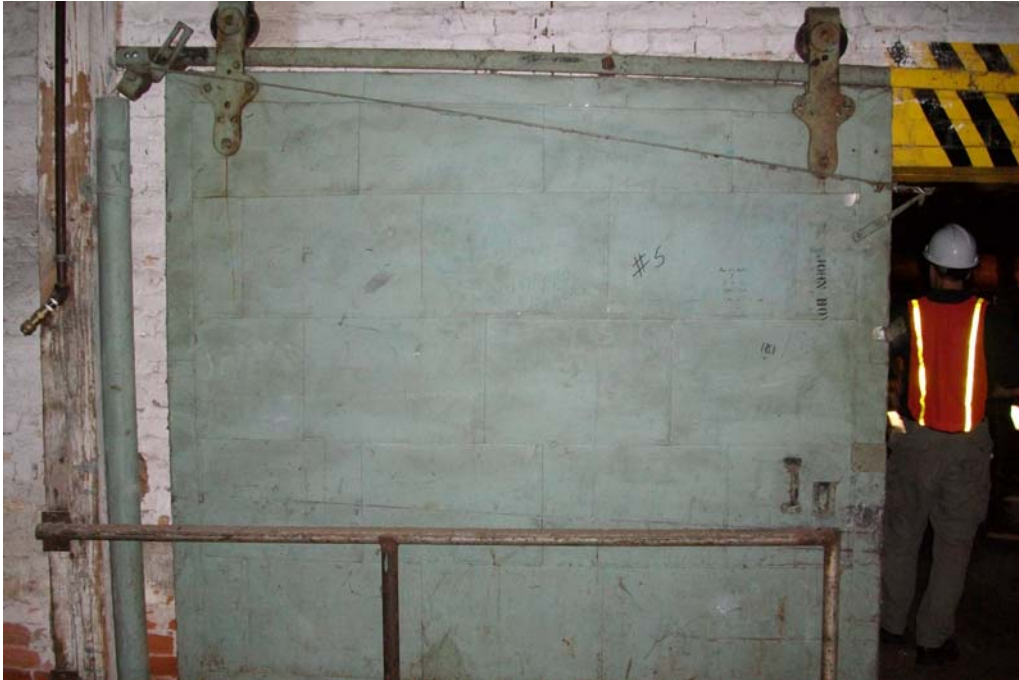
Photograph No. 5: Typical sliding track, wooden doors with pressed metal finish in Warehouse No. 5.
