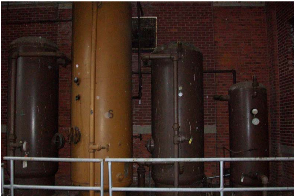
Photograph No. 6: Compressor tanks.
