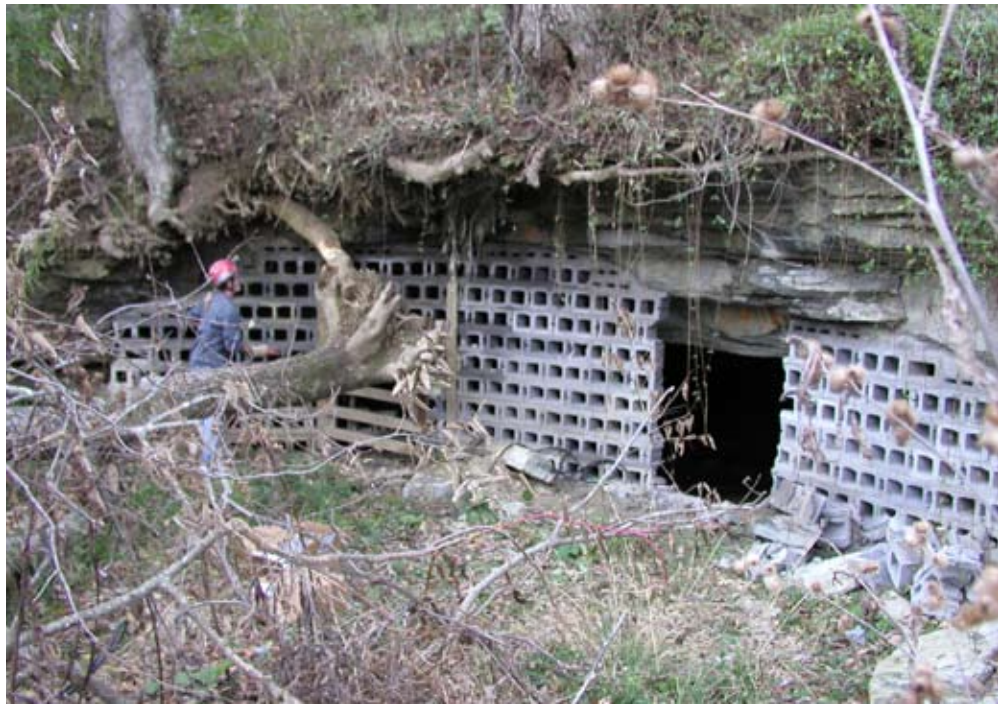
The cinder block wall failed to keep out trespassers; it was replaced with a “bat-friendly” steel gate below. Brent Harrel, USFWS photo
