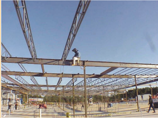
A steel worker at a Denark Construction jobsite secures himself to a beam. Denark requires fall protection for all workers operating more than six feet above ground.
