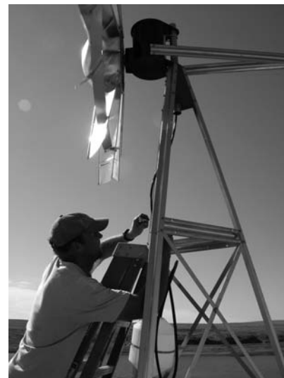
Miles City Field Office Fishery Biologist Joe Platz makes adjustments to an aeration windmill being installed at Homestead Reservoir Oct. 5. The windmill is the fourth such project in Prairie County designed to improve fish habitat on BLM-administered lands.
