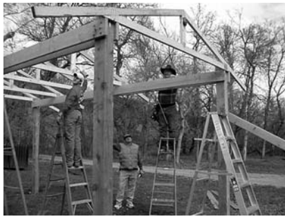
Volunteers construct a shelter at Alkali Creek Horse Camp. Photo by Dennis Bucher
