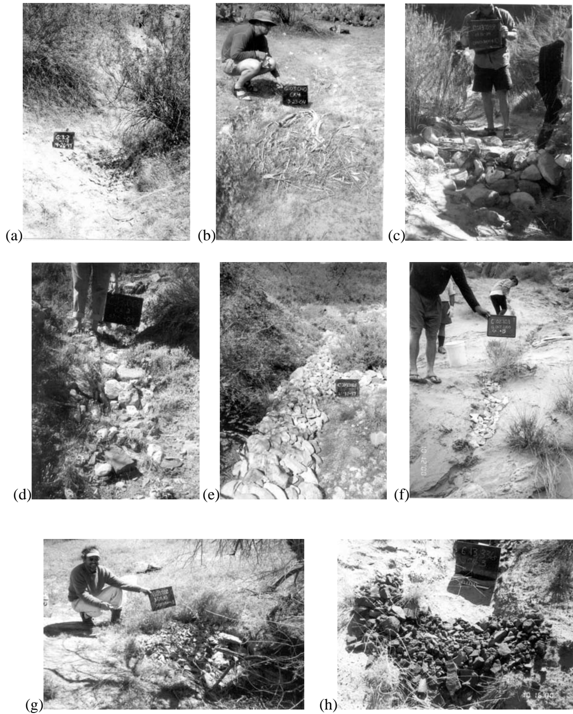
Figure 10. Checkdam types constructed along the Colorado River corridor. (a) brush and rock lining (b) brush lining (c) brush and rock checkdam (d) rock lining (e) water diversion bar (f) knickpoint treatment (g) headcut and (h) rock checkdam.
