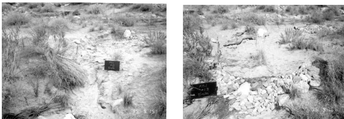
Figure 5. Location of a checkdam before and after construction on the Palisades Delta in 1995.
