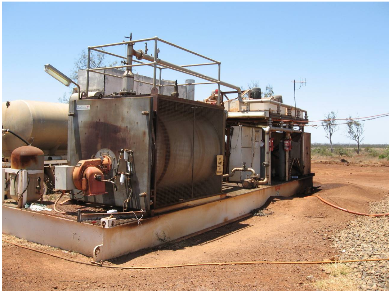
Figure 9.—Tomlinson boiler for inertization at an Australian coal mine.
