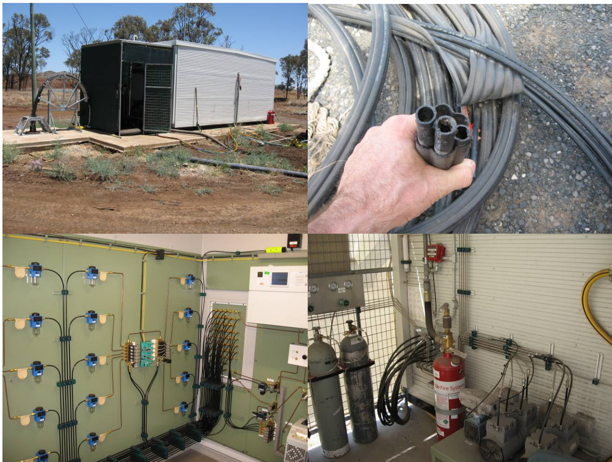
Figure 8.—Continuous atmospheric gas monitoring system in Australia. Top left: Monitoring shed over mine showing borehole and sample tubes. Top right: Close-up of sample tube bundle. Bottom right: Sample tube pumps. Bottom left: Inside monitoring shed showing manifold and gas analyzer.
