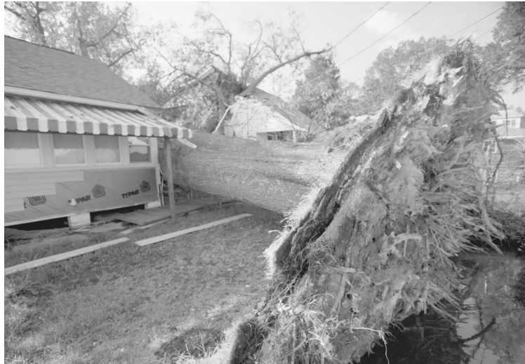
This uprooted tree in Colonial Beach is one of thousands of trees downed by Hurricane Isabel throughout the Commonwealth of Virginia. FEMA photo by Andrea Booher
