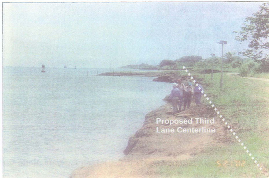
Figure D-1-2 Standing Along North Shoreline, Looking North Toward The Atlantic Approach. Proposed Third Lane Centerline Depicted
