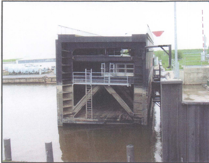
Figure B-2-6 Spare Rolling Gate in Mooring Location
