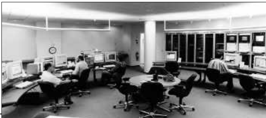
← The newly completed APS Main Control Room (MCR). This photo was taken during the afternoon shift on March 23. (ANL photograph 19366K #12A)
