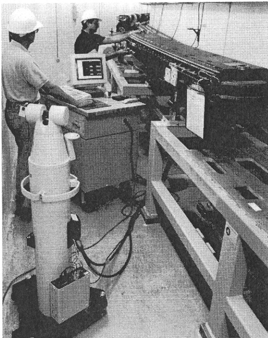
↑ Bldg. 415/Booster Bldg. — Installation of the booster synchrotron continues. Jaromir Penicka (l.) and Joe Error (both ASD-Survey & Alignment) use a laser tracker to align synchrotron magnets to within \pm 50 microns.
