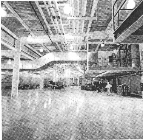
↑ Bldg. 420/Rf/Extraction Bldg. — Beneficial occupancy of the Rf/Extraction building was granted to the Project on May 18, clearing the way for installation of rf equipment.
