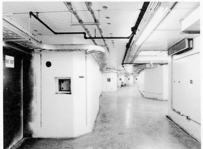
↓ ALD/PD Milestone #27 — The completed interior of the APS Storage Ring Tunnel at Zone #1 adjacent to the Early Assembly Area.
