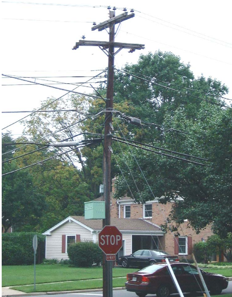
Figure D-20: Site B power lines as viewed from the measurement vehicle located at Point C
