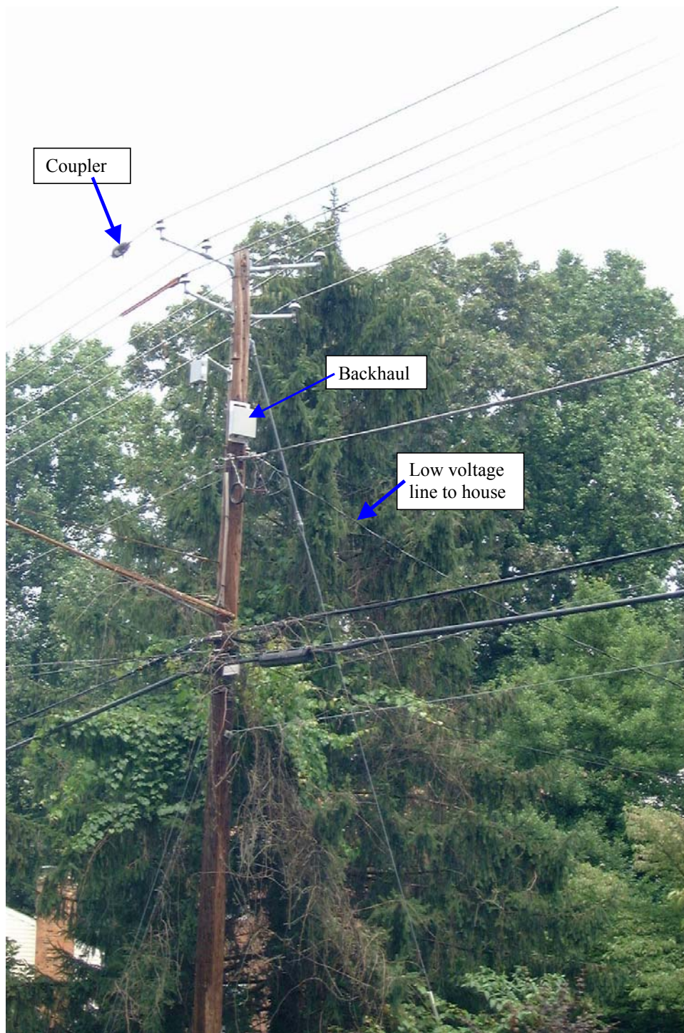
Figure D-41: Measurement Site H utility lines located immediately in front of house as viewed from across the street parallel to the approximate location of the measurement vehicle.
