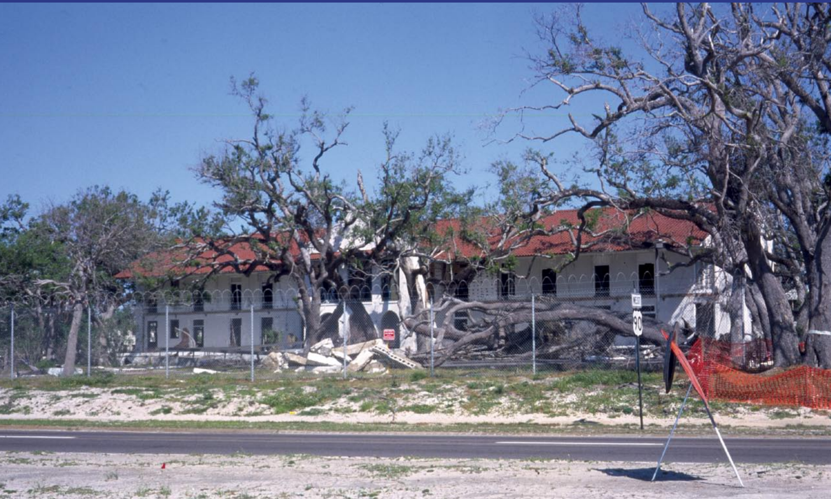
Veterans Administration Hospital, Gulfport, MS after Hurricane Katrina
