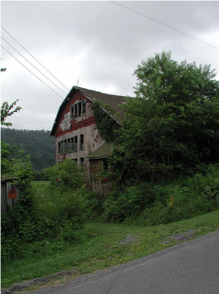
097-LM-002-03. Barn gable. Lower Mahanoy Township, Northumberland County. An extreme example of converting a barn to poultry use.
