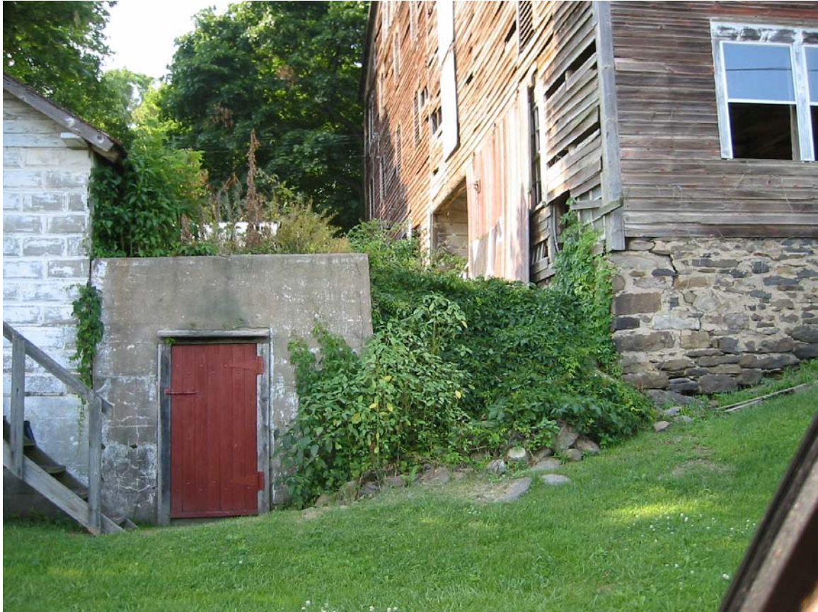
037-NC-006. Root cellar between barn and ice house, North Center Township, Columbia County.
