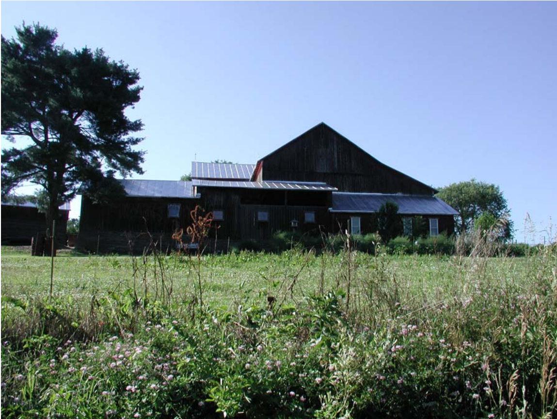
037-gr-008-07. Barn south side. Greenwood Township, Columbia County. Essentially, the outbuildings are grafted onto the main barn.
