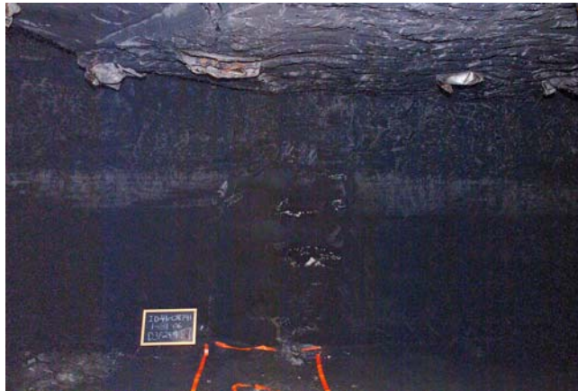
Figure 24 - Post-Explosion Location of Seal No. 5
