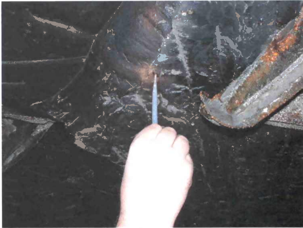
Figure 3. Collection of water droplets on the roof and fracture faces where "blue haze" was observed between spads 3986 and 3981.
