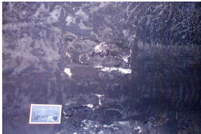
Figure 22 - Post-Explosion Location of Seal No. 3
