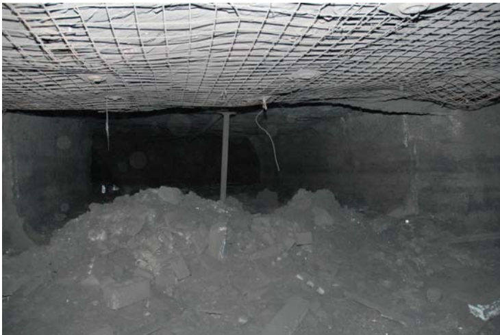
Figure 6 - Damaged Stopping at 59 Crosscut, No. 4 Belt
