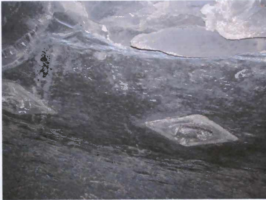
Figure 2. Two sets of paired, linear ridges define an acute angle in the roof horizon just inby spad 4010. R. J. Lee sample collection effort on March 1, 2006 extracted samples of this feature. In this photo, the linear feature is truncated by a shallow stress pot-out.
