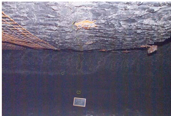
Figure 26 - Post Explosion Location of Seal No. 7
