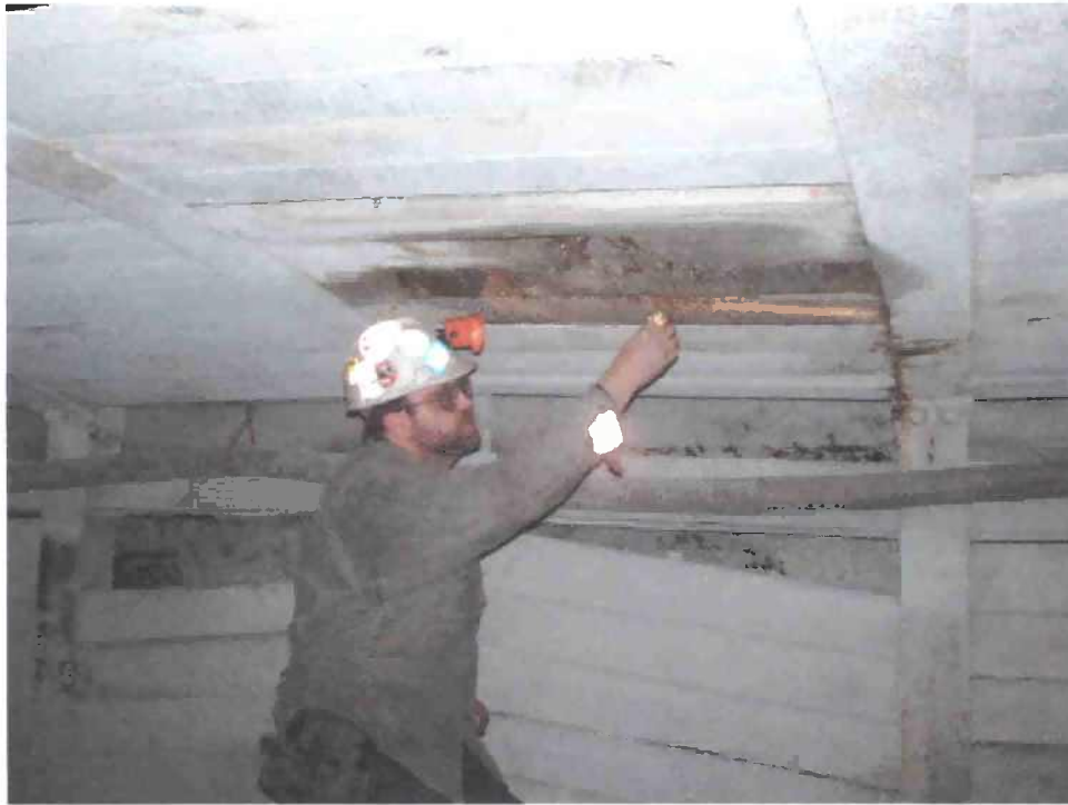
Figure 1. Collection of dripping water in the track entry of the Main, between Crosscuts 32-33.
