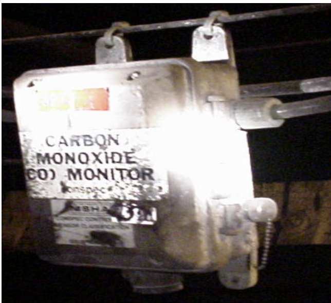
Example carbon monoxide sensor installation
