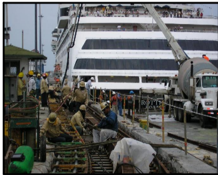
Method for conducting locks maintenance while the lane remains open to traffic. Note the passenger vessel being immediately followed by a concrete pouring barge.
