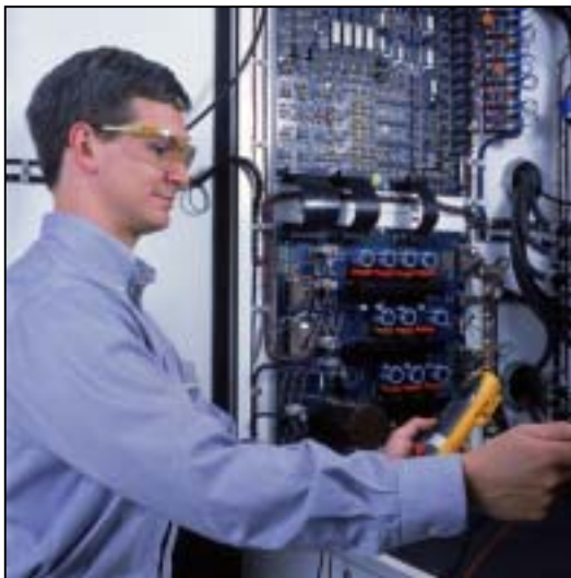
A researcher measures inside a 100-kW inverter
