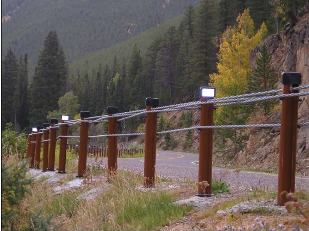
Figure B.2: High Tension Cable, HTC
