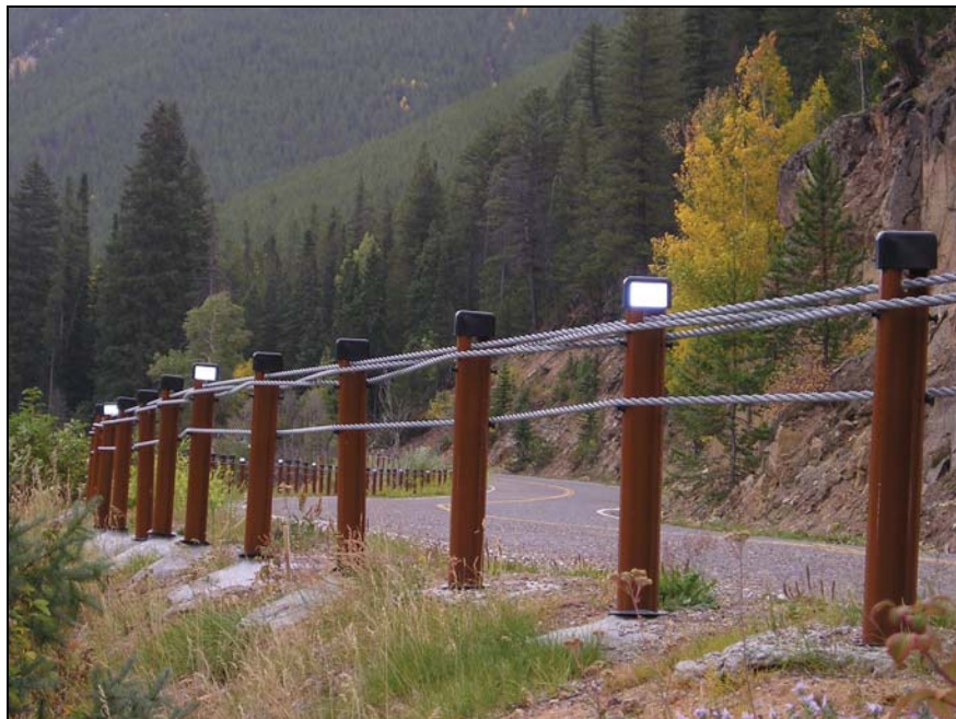
Figure 3.2: High-Tension Cable, HTC
