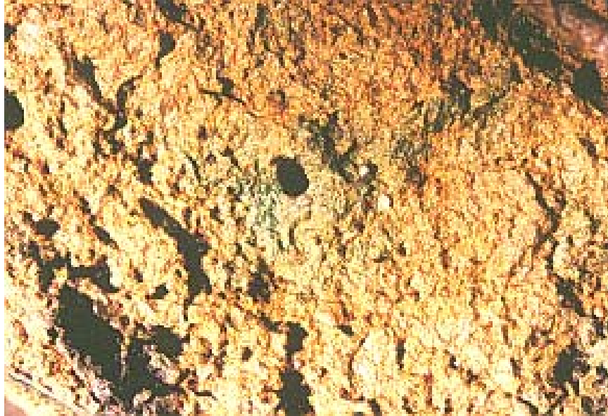
Figure C-9.0-2. Earthworm hole in barrier soil layer
