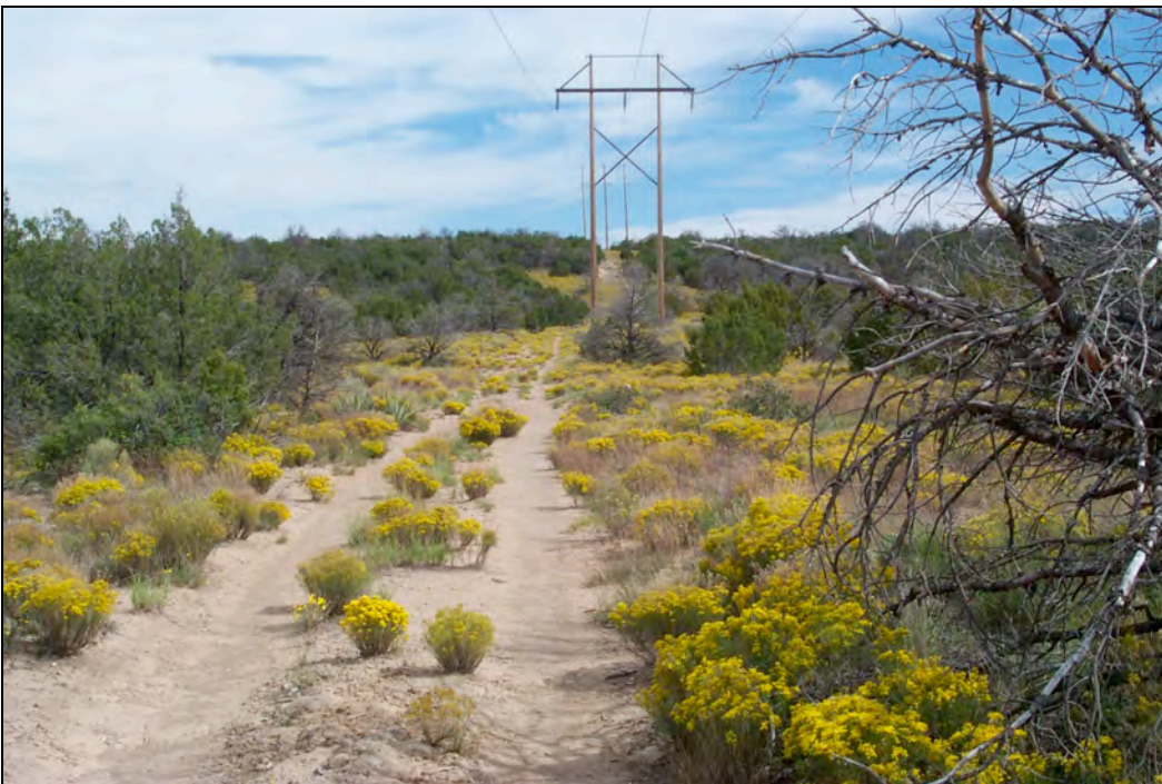
Figure 5. Erosion occurring along a power line road.
