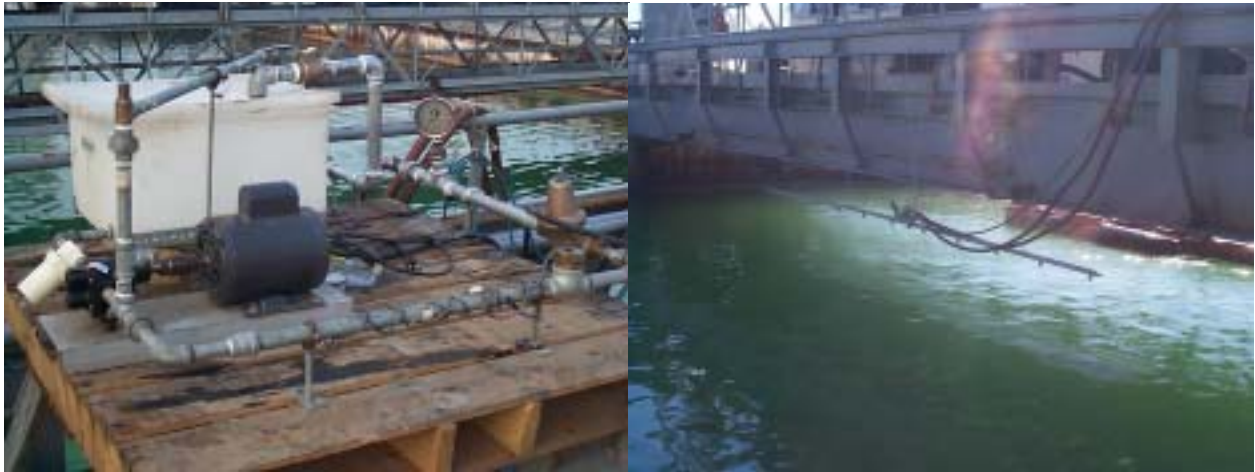
Figure 5. Dispersant Supply Tank and Pump and Dispersant Spray Bar in Operation
