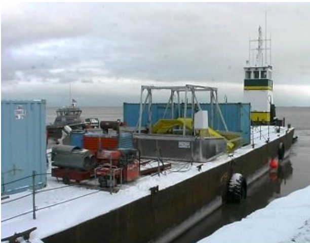
Work platform and Lifting Grated Belt put together on barge. Auxiliary equipment (hydraulic power pack, air heater, water pumps, electric generator, hot water pressure washer) is also stored on board.
