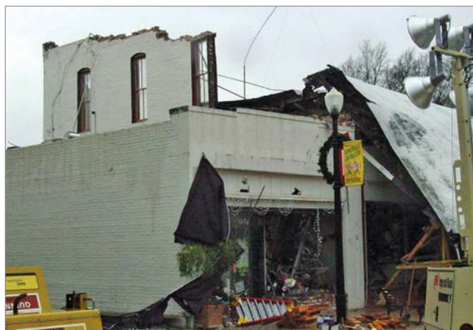
Collapsed roof in downtown Paso Robles following the San Simeon earthquake of December 22, 2003. Two people were killed by falling debris when they ran out of the building. (USGS photo)
