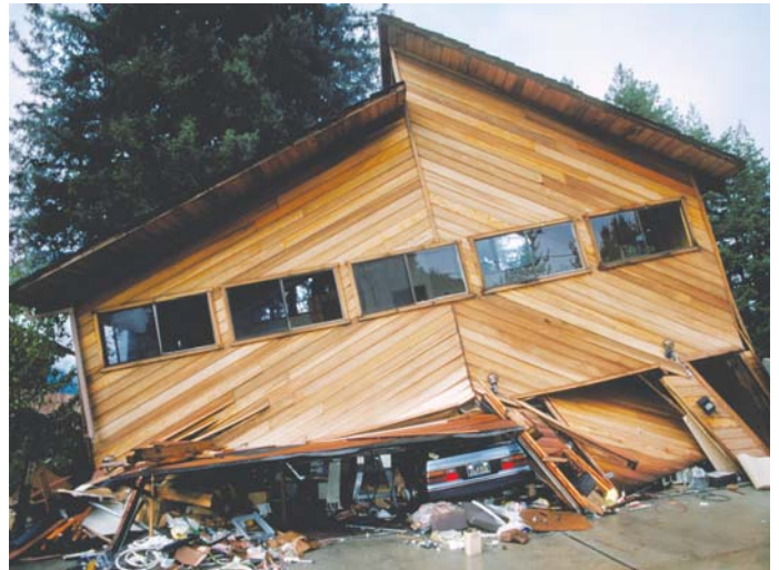
This home in the Santa Cruz Mountains collapsed in the 1989 magnitude 6.9 Loma Prieta earthquake (USGS photo).
