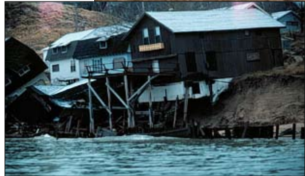
High lake levels on Lake Michigan in 1986 caused severe erosion.
