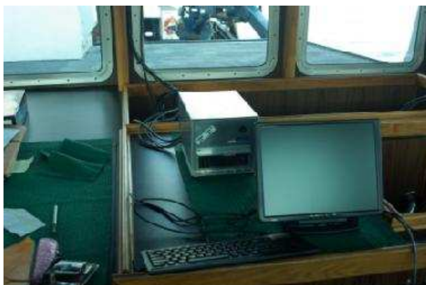
Figure A1. EM control box and user interface installations on two different vessels.
