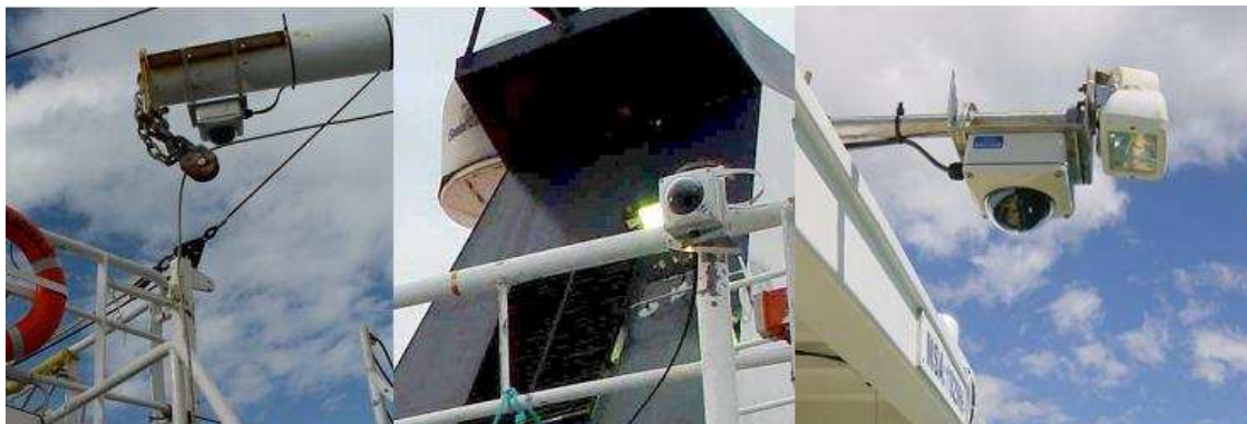
Figure A2 CCTV camera installations on three different fishing vessels. Each camera has a mounting bracket and stainless steel mounting straps.
