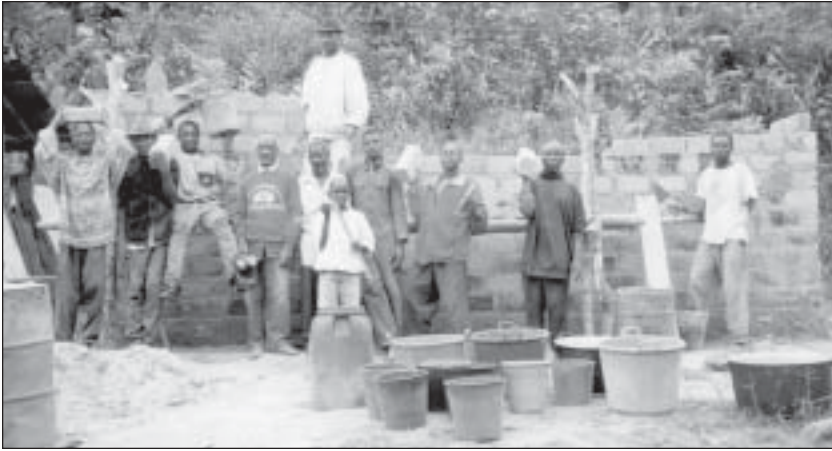
SPA funds helped purchase supplies for this school construction project in Gabon.
