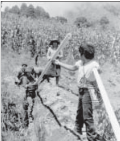
Communities often contribute transportation and labor while SPA and other sources fund the purchase of pipes or pumps.
