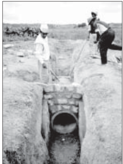
A drainage system is constructed with the support of a municipality in Madagascar.
