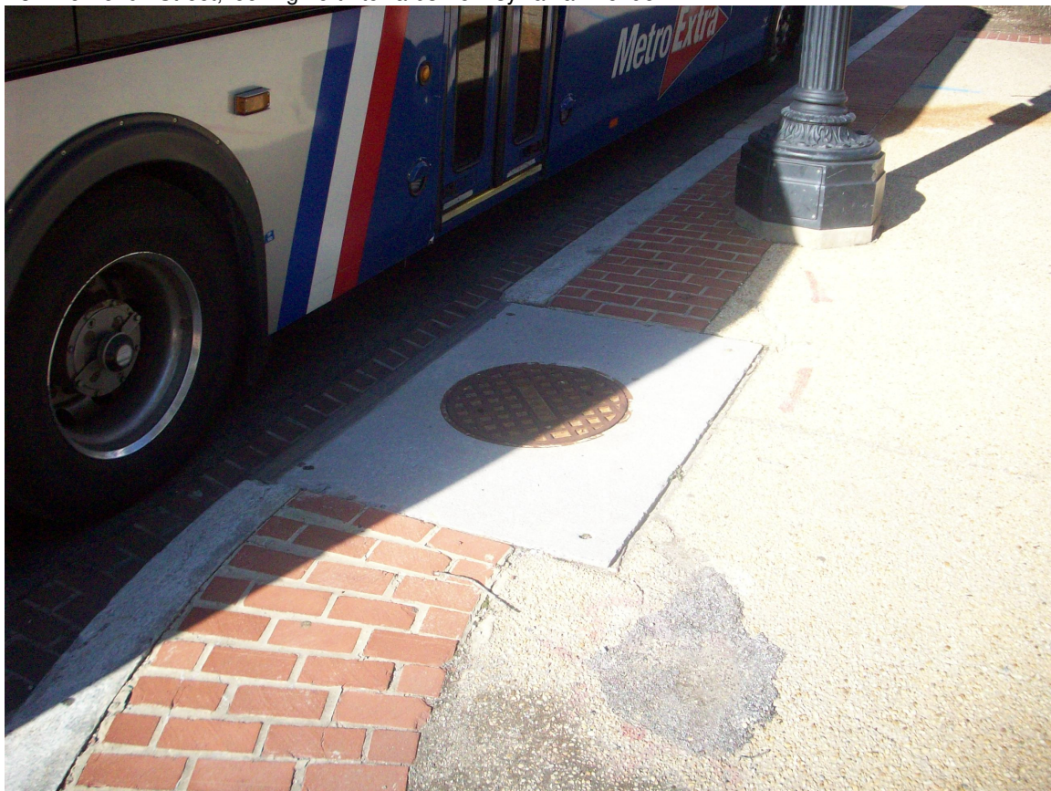
16. View of a stormwater drain, located approximately 15 feet north of the 9 th Street entrance.
