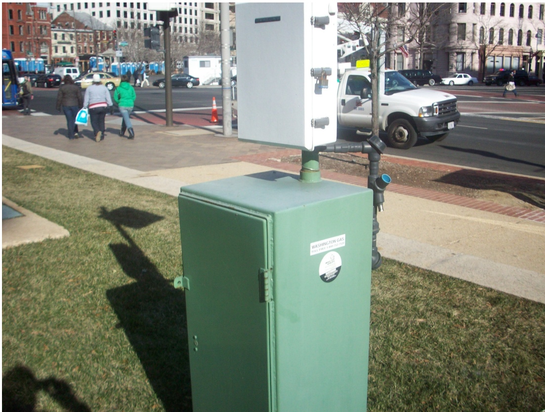
11. View of a Washington Gas line, located approximately 30 feet north of the 7 th Street entrance.
