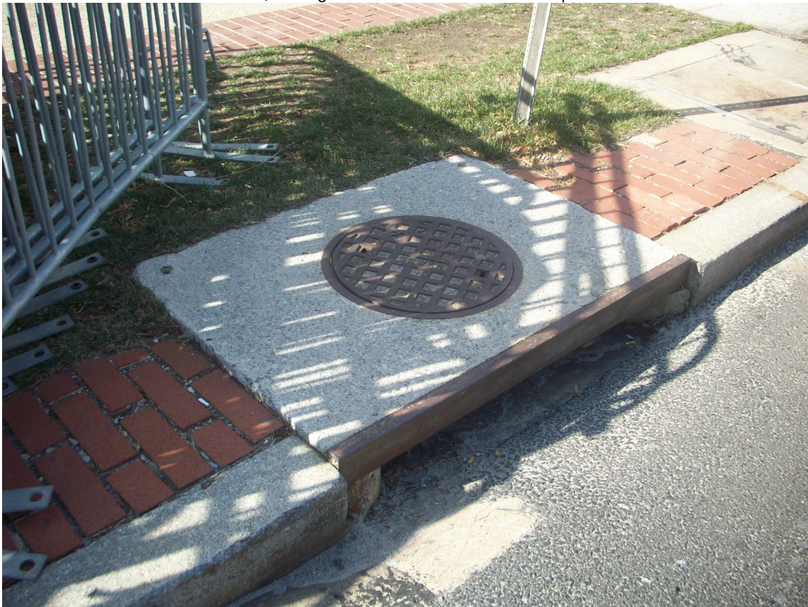
10. View of a stormwater drain, located on 7 th Street, approximately 25 feet from the 7 th Street entrance.
