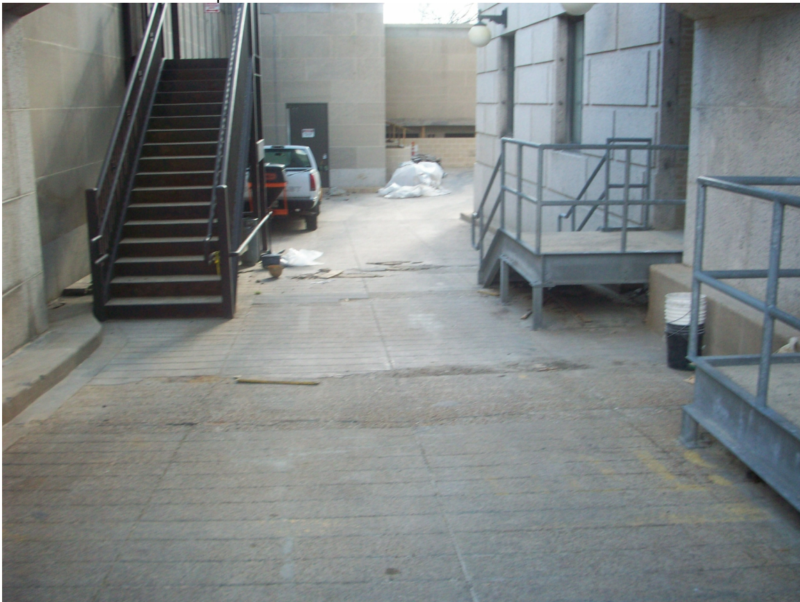
8. View of the southern portion of the 7 th Street entrance moat area.
