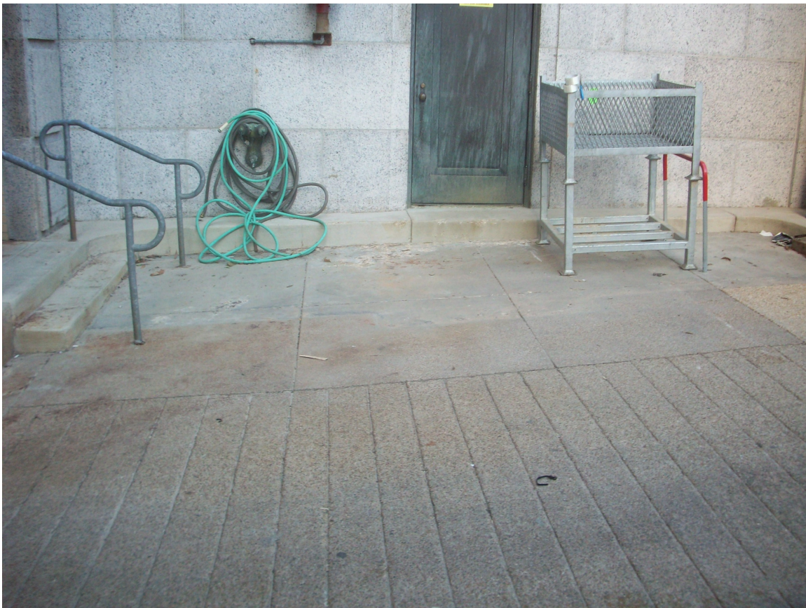
7. View of the northern portion of the 7 th Street entrance moat area.
