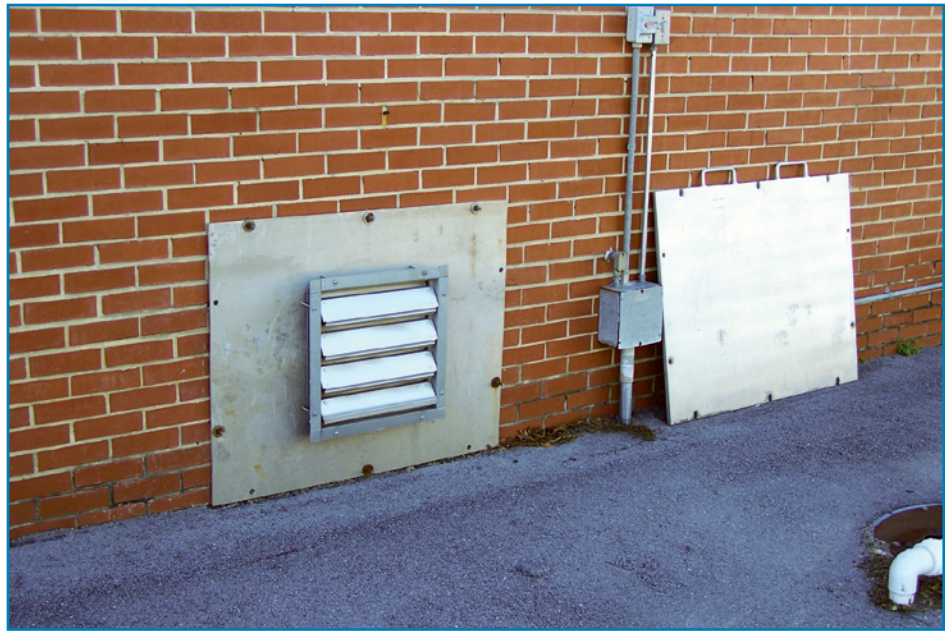
Figure 3-44: The ventilation openings for the original building's crawlspace are protected with floodproofing panels that are bolted in place when flooding is predicted.
