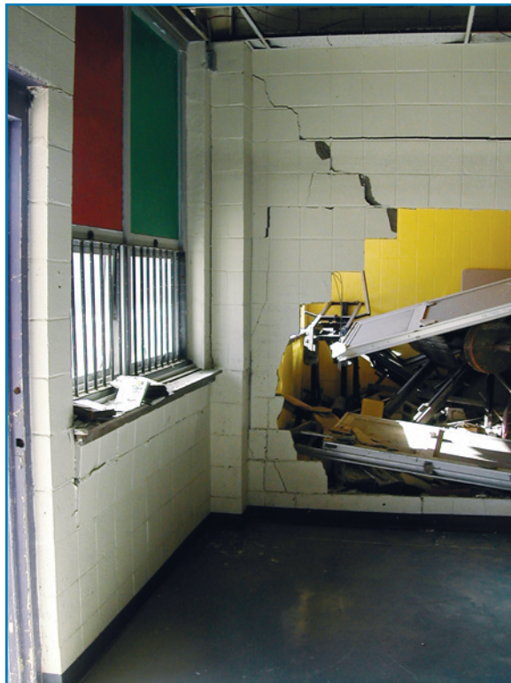
Figure 3-14: Interior unreinforced masonry walls of the Port Sulphur High School in Louisiana were damaged by hydrostatic loads associated with Hurricane Katrina's storm surge (2005).
