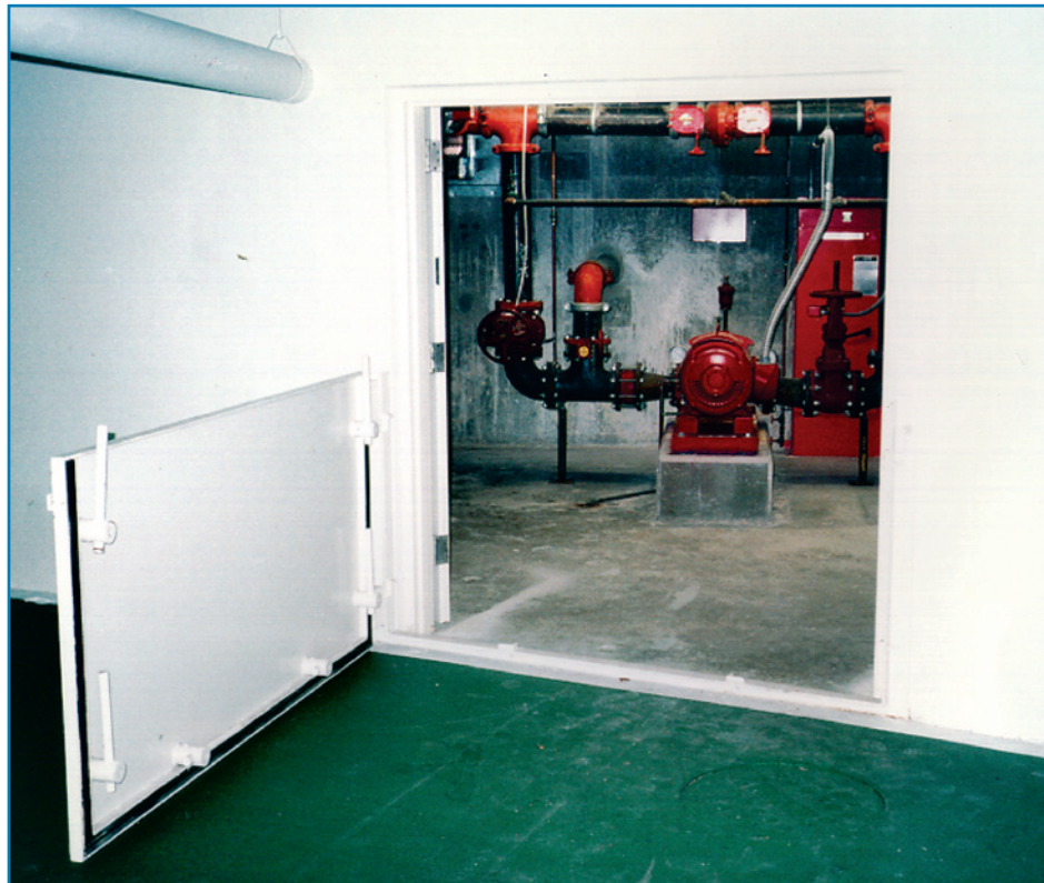
Figure 3-38: Equipment room with watertight door SOURCE: PRESRAY CORPORATION
