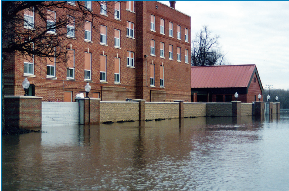
Figure 3-39: A masonry floodwall with multiple engineered openings in Fargo, ND during flooding in 2001.
