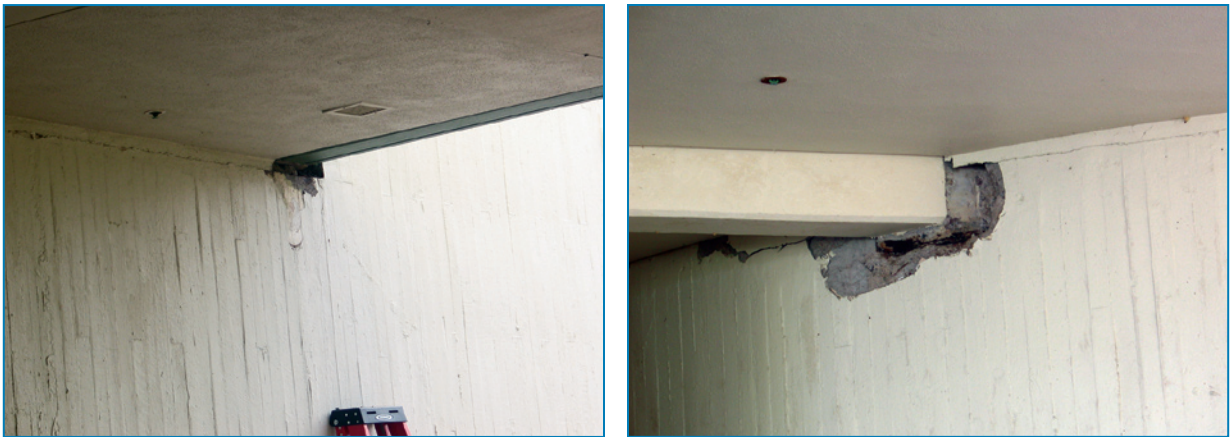
Figure 2-40: Spalling at beam connections
