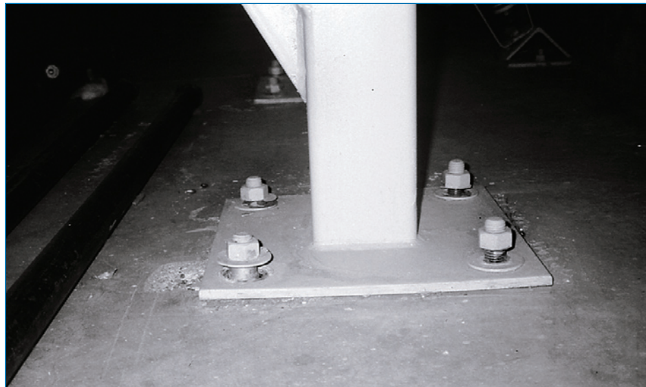
Figure 2-32: Anchor bolts stretched by large seismic accelerations at roof level
