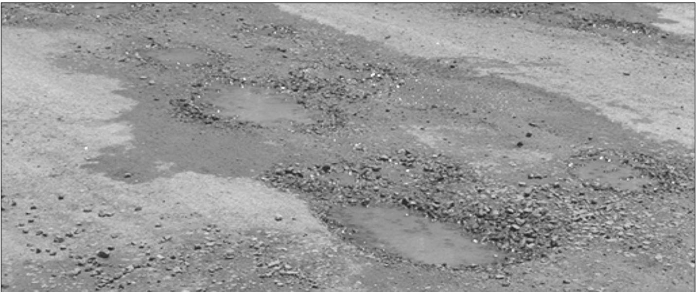
Potholes in Road Base
