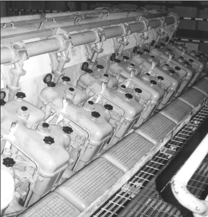
Diesel Power Generator, Marshalls Energy Company
