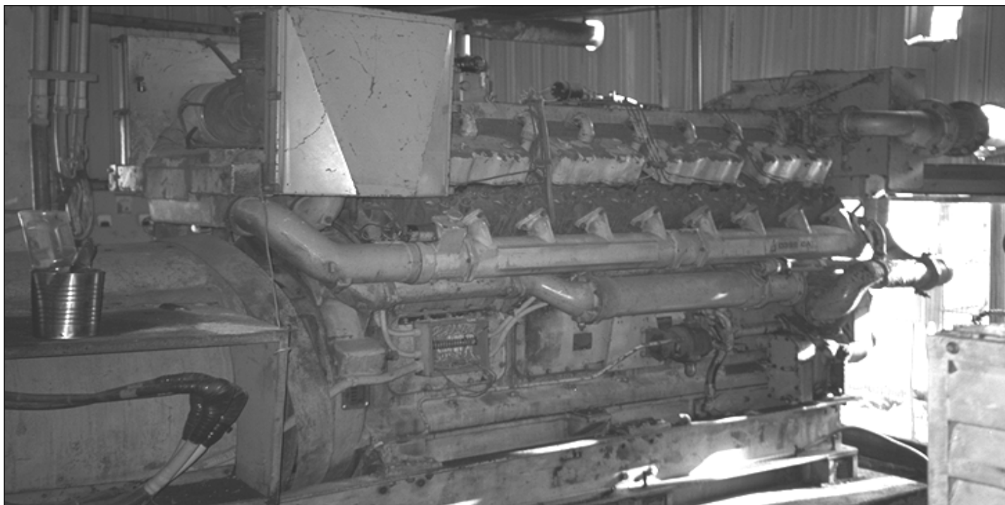
Diesel Power Generator on Tonoas, Chuuk, Chuuk Public Utility Corporation, FSM
