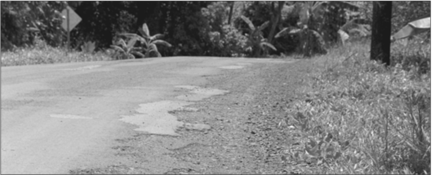
Eroded Asphalt Shoulder
