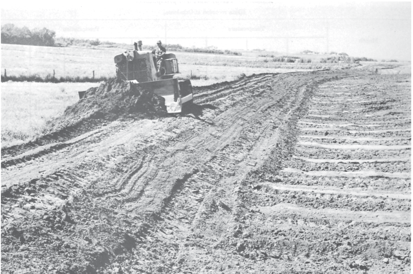
Figure 31.—Construction of a diversion terrace on Radford silt loam to protect it from damage caused by runoff.
