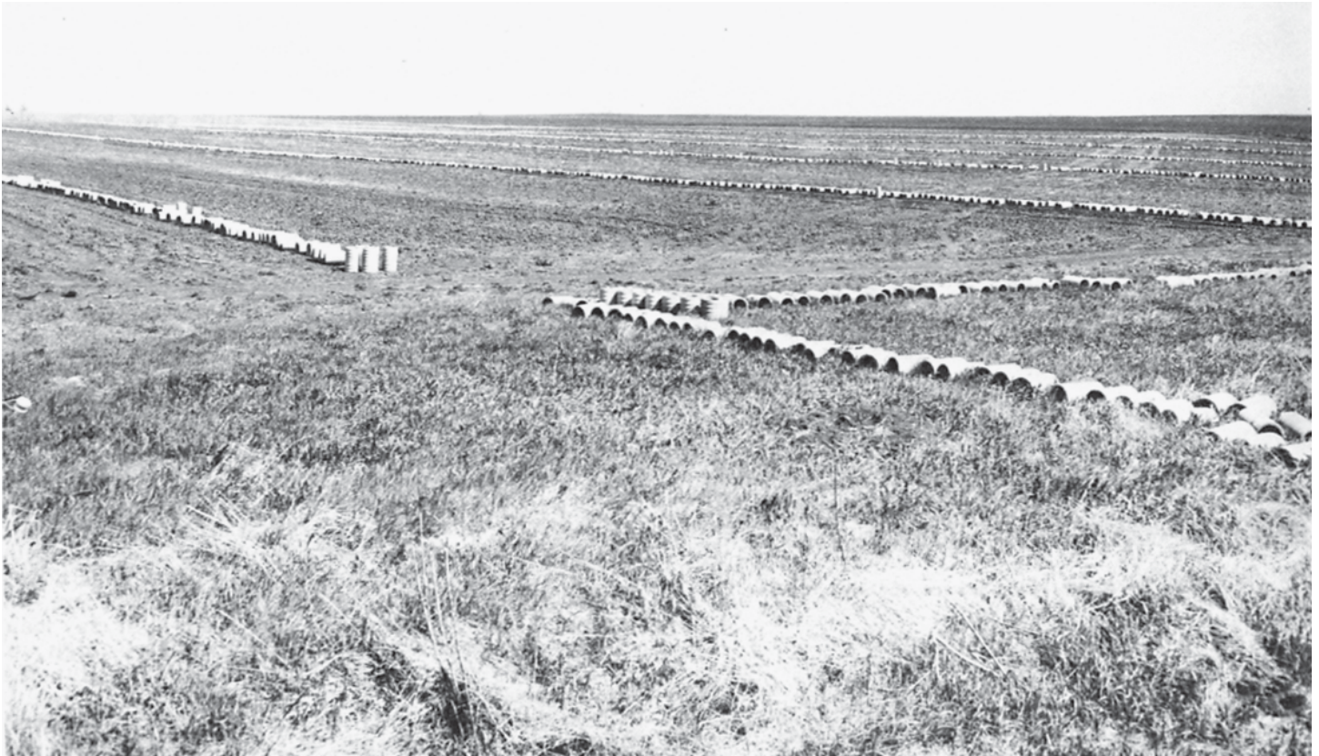
Figure 10. —Drainage tile ready for installation on Sawmill-Garwin silty clay loams. Muscatine and Tama soils are in the background.
