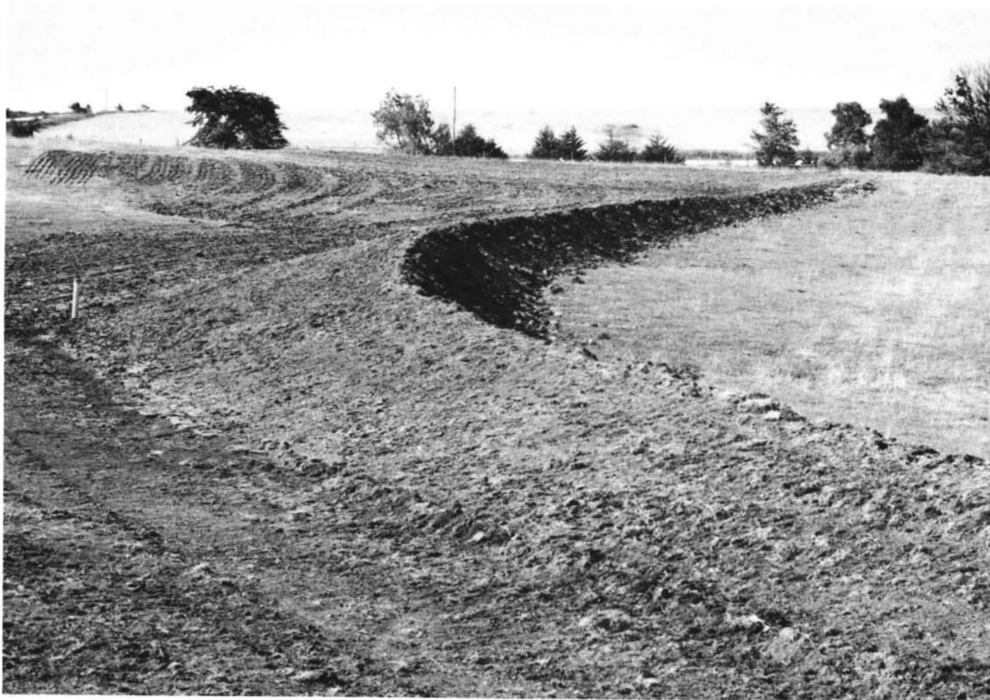
Figure 16.—A tile outlet terrace with a steep back slope helps to control water erosion on Nira silty clay loam, 5 to 9 percent slopes, moderately eroded.
