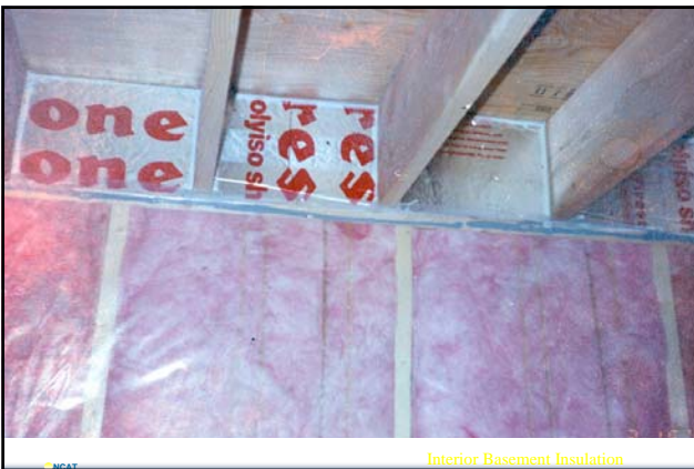
Interior Basement Insulation
