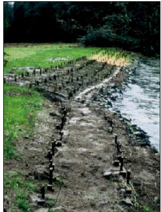
Mill Creek – February 1998 After Installation of Live Fascines (foreground), Brush Mattress, and Live Stakes with Erosion Control Fabric
