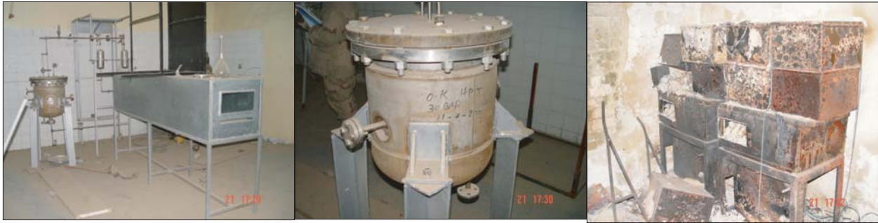
Building 59: Reverse osmosis laboratory (R29) (left and center); burnt metal cases (R31) (right).
