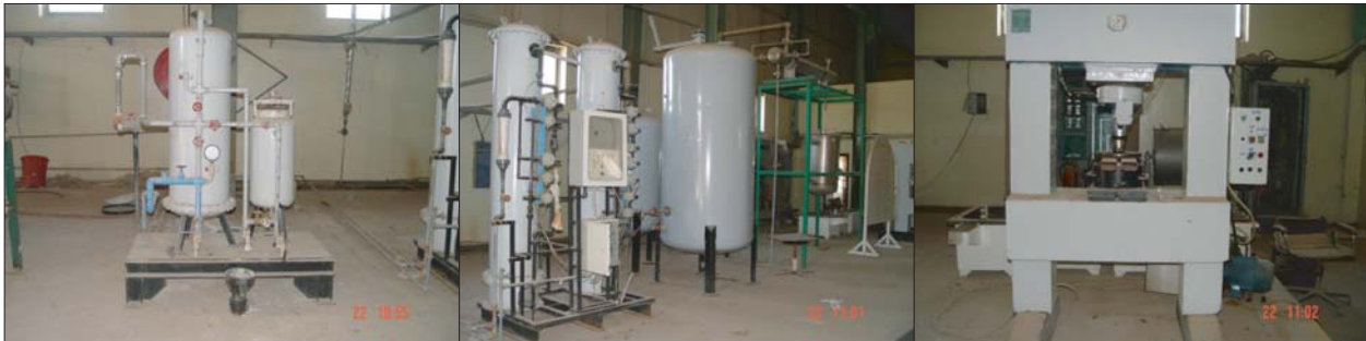
Building 53, Room 1. Water-processing system (left and center); press (right).
