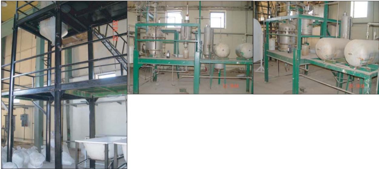
Building 53, Room 1. Bathtubs and dryer (left); clove oil production equipment (center and right).
