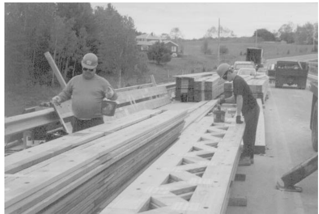
Figure 6—Galvanized metal plate connectors of each truss were brush-painted at the site for additional protection from corrosion.
