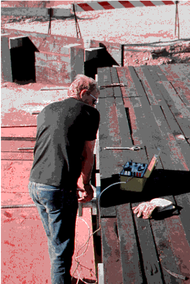
Figure 11—Measuring bar force data with a portable strain gage indicator and load cell.
