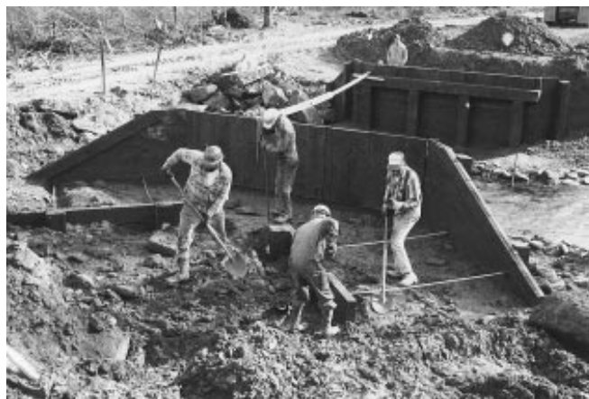
Figure 5—Construction of the post and sill abutments for the Little Salmon Creek bridge.
