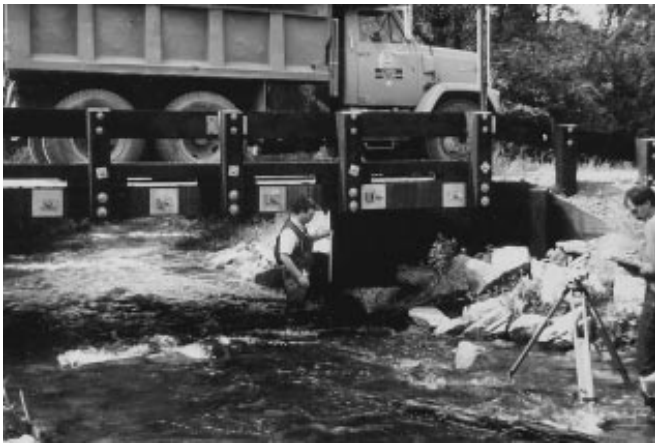
Figure 13—Load test 1 bridge deflections were measured by suspending a calibrated rule from the deck underside and reading displacement values with a surveyor's level.
