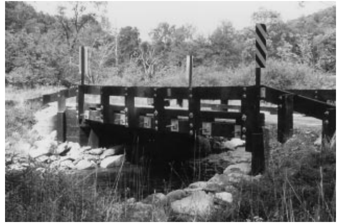
Figure 18—The 2.5 in. of superstructure sag on the downstream bridge side is visually evident in the bridge deck and the railing.
