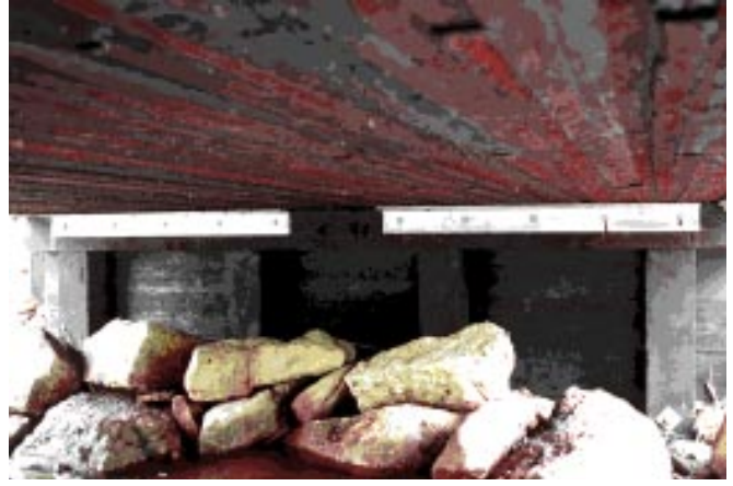
Figure 9 —Attachment of the superstructure was by bolting the deck to steel angles that were then bolted to the side of the substructure cap.
