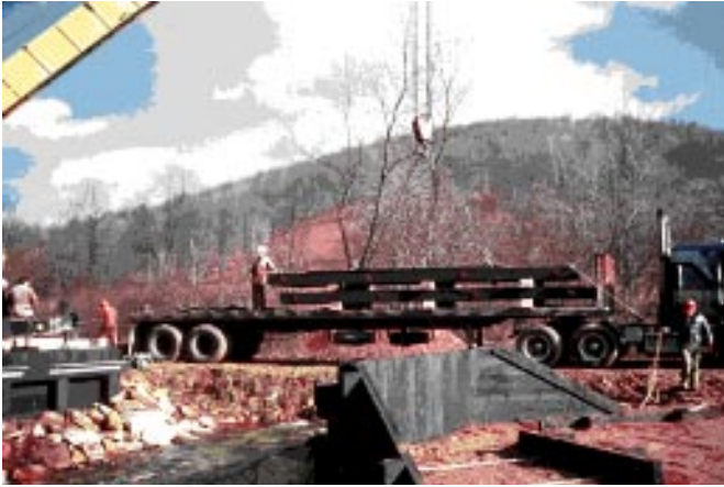
Figure 6 —The two deck sections for the Little Salmon Creek bridge were transported from the treating plant to the bridge site on a flatbed truck.
