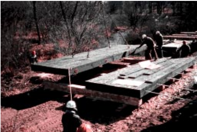
Figure 7 —At the bridge site, the temporary steel bars in the two deck sections were removed and stressing bars were inserted through both deck sections.
