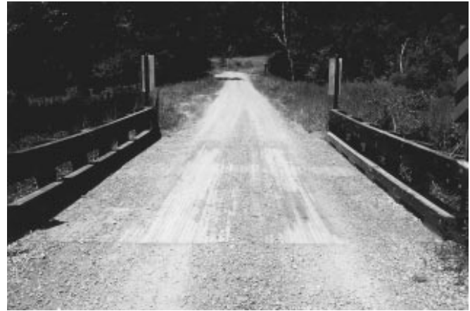
Figure 25—Debris accumulations on the bridge's deck noted during condition assessment.
