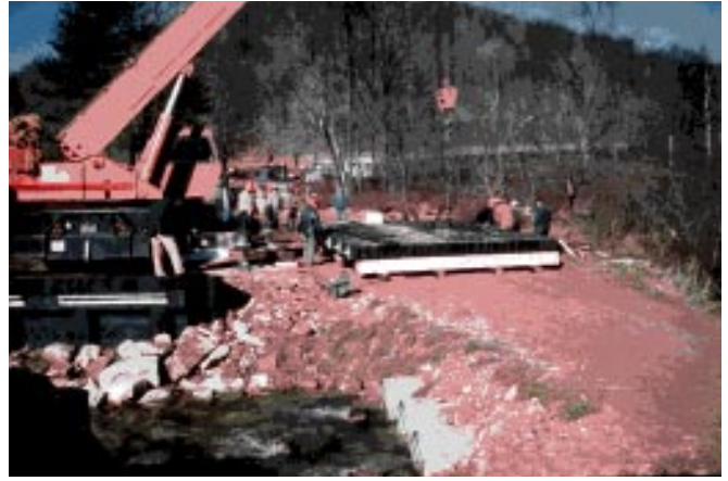
Figure 8 —After the stressing bars were tensioned, the entire superstructure was lifted on the abutments by a small crane.
