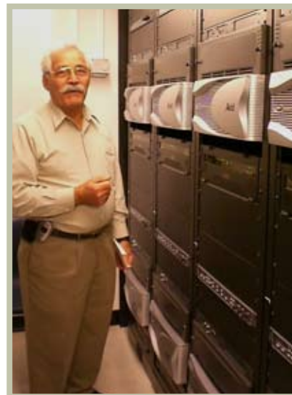
Chief Engineer Alex Cusati stands in front of the equipment used to support Committee broadcasts.
