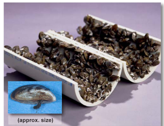
The small zebra mussels densely colonize inside cooling water intake pipes of power plants thus leading to significant power outages and expense.
