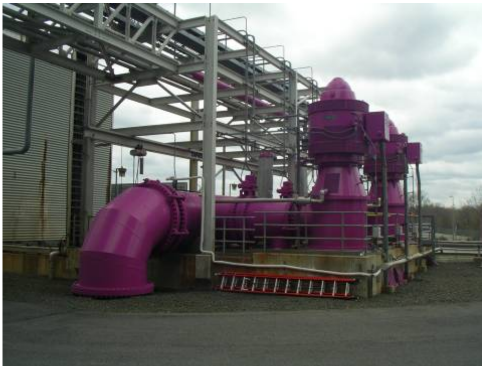
Figure 7 – Reclaimed Water Pipe and Recirculating Pumps (Source: Veil 2007)
