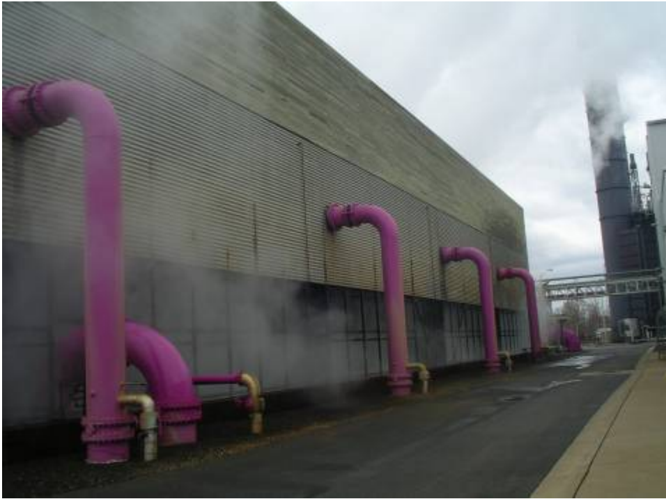
Figure 6 – Reclaimed Water Lines and Cooling Tower (Source: Veil 2007)
