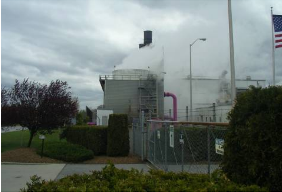
Figure 8 – Cooling Tower Plume (Source: Veil 2007)
